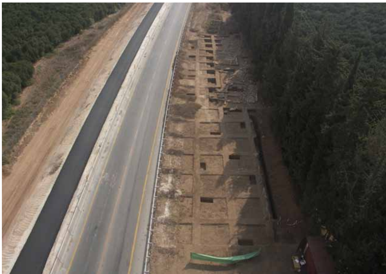
Fig. 2.2. General view of Area B (looking east), with Area Ba in the foreground. This section of the site was found to be devoid of artifacts and archaeological remains. Notice the deep test channel on the south side of the area (in the right foreground).
