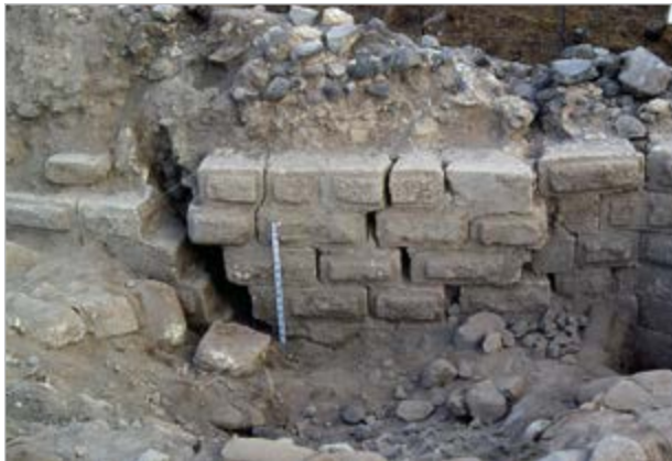
Figure 18.4. The displacement along the northern wall of the fortress. The amount of displacement is identical to that measured along the southern wall.
